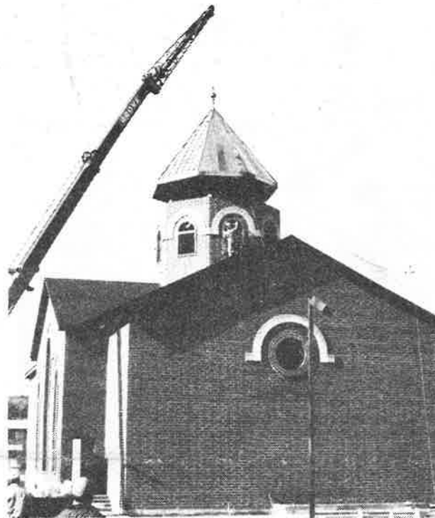
A dramatic moment! The cone of the dome is being placed by a huge crane.
