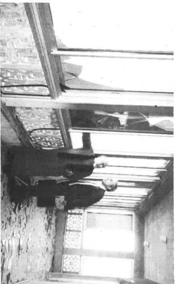
His Holiness and Dr. Vazken Der Kaloustian, a member of the Central Executive Council, inspect the damage to the Catholicate complex from the upper floor of the Veharan (Catholicos' residence).
